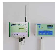
Installation together with Powerbox
